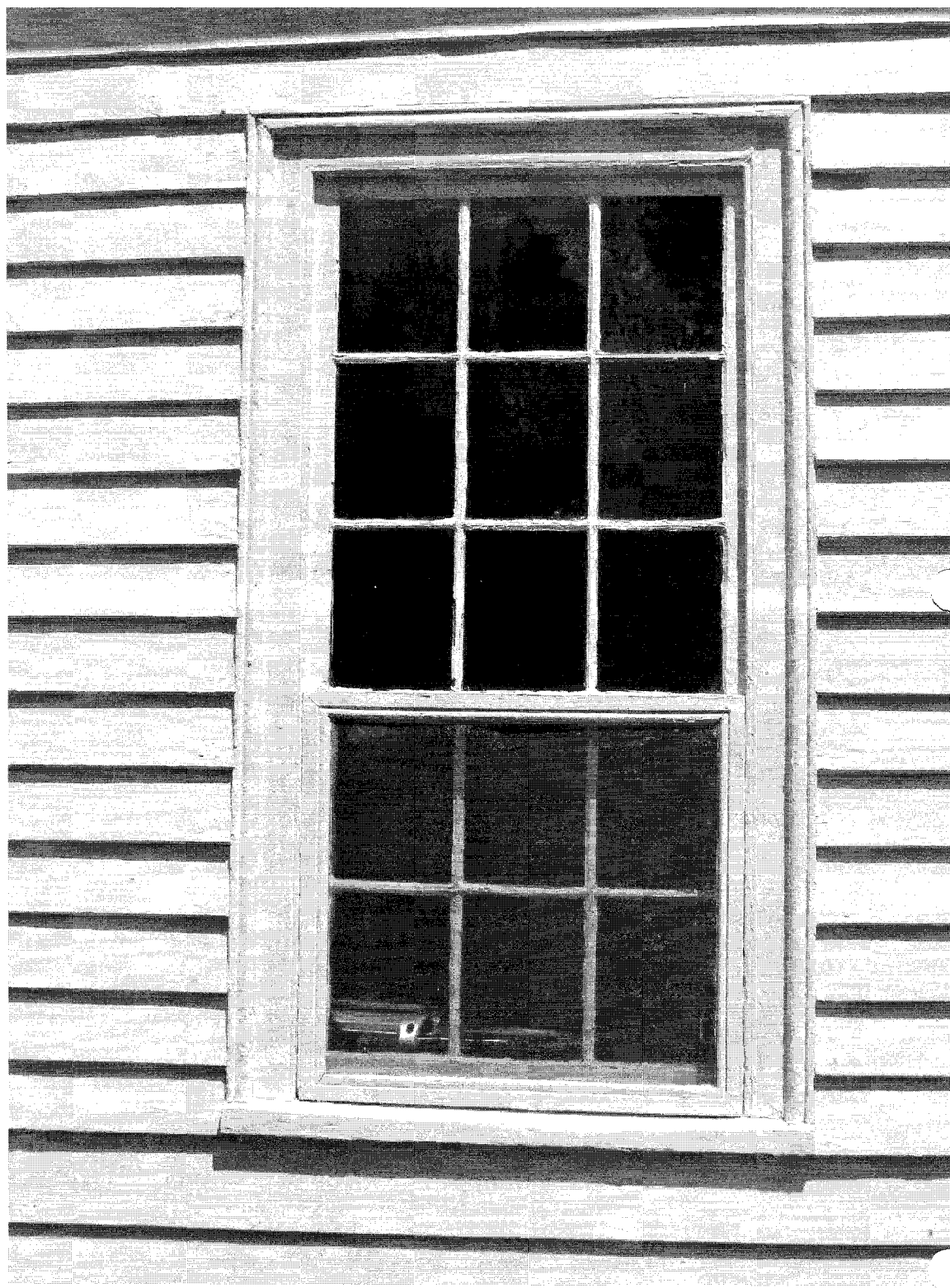
The photo on this page shows the simple trim of a window from the Cape style period with 9 over 6 window panes. In the next issue we will be looking at the Greek Revival/ Italianate Transitional period from c. 1850 to 1890. In these homes doors and windows became more ornate.
